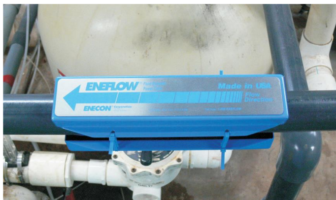
Figure 1: ENEFLOW magnet installed in the water way.
